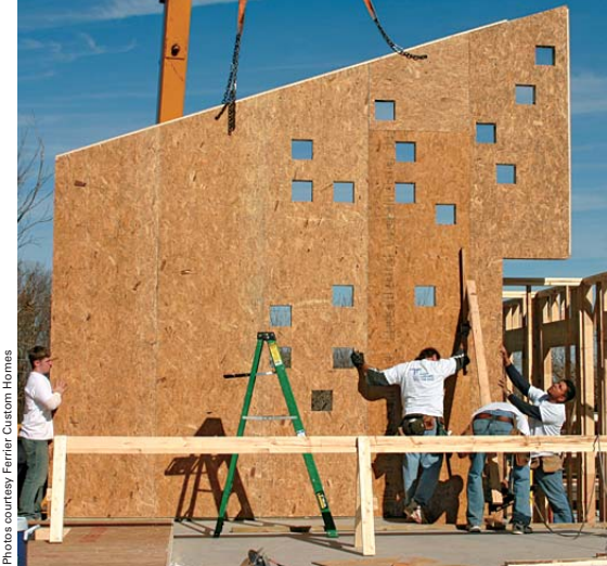
LEFT: A precast structural insulated panel is lowered into place. FAR LEFT: Heather Ferrier in her award-winning home.
